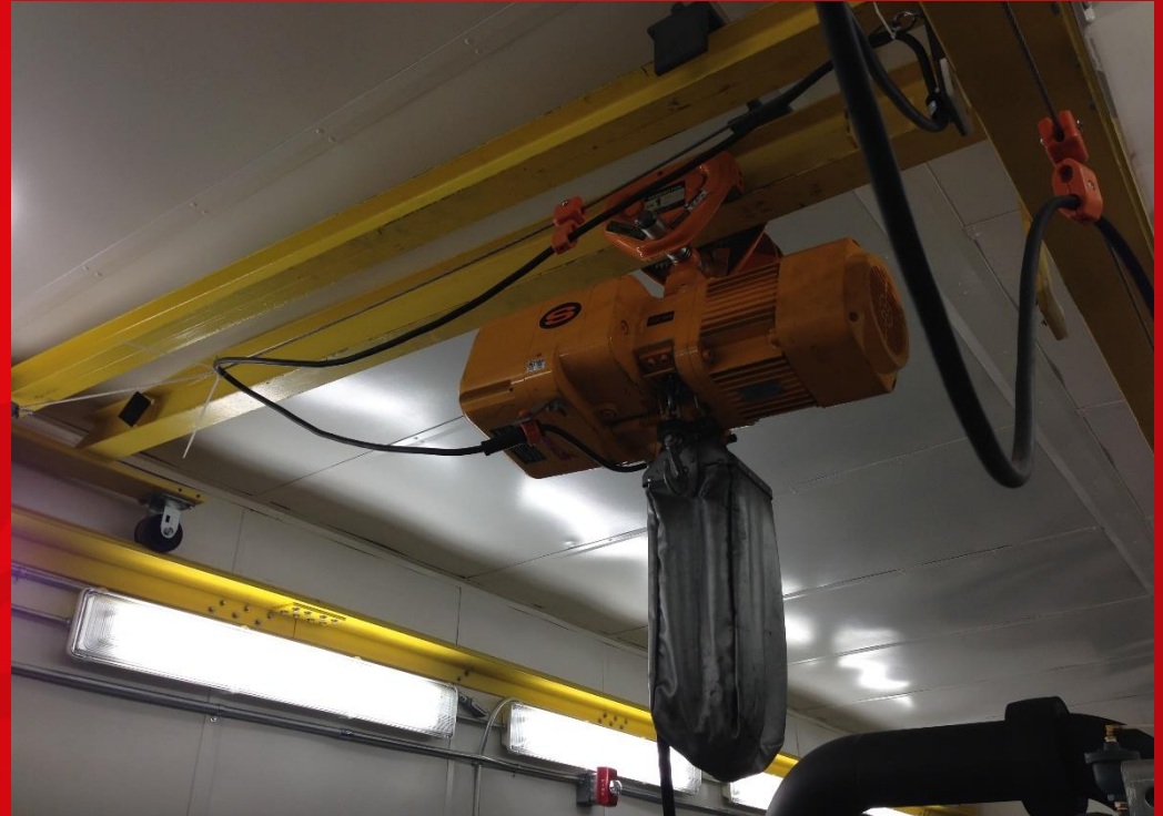
Existing gantry and hoist system in the Chiller 3 Testing Room
